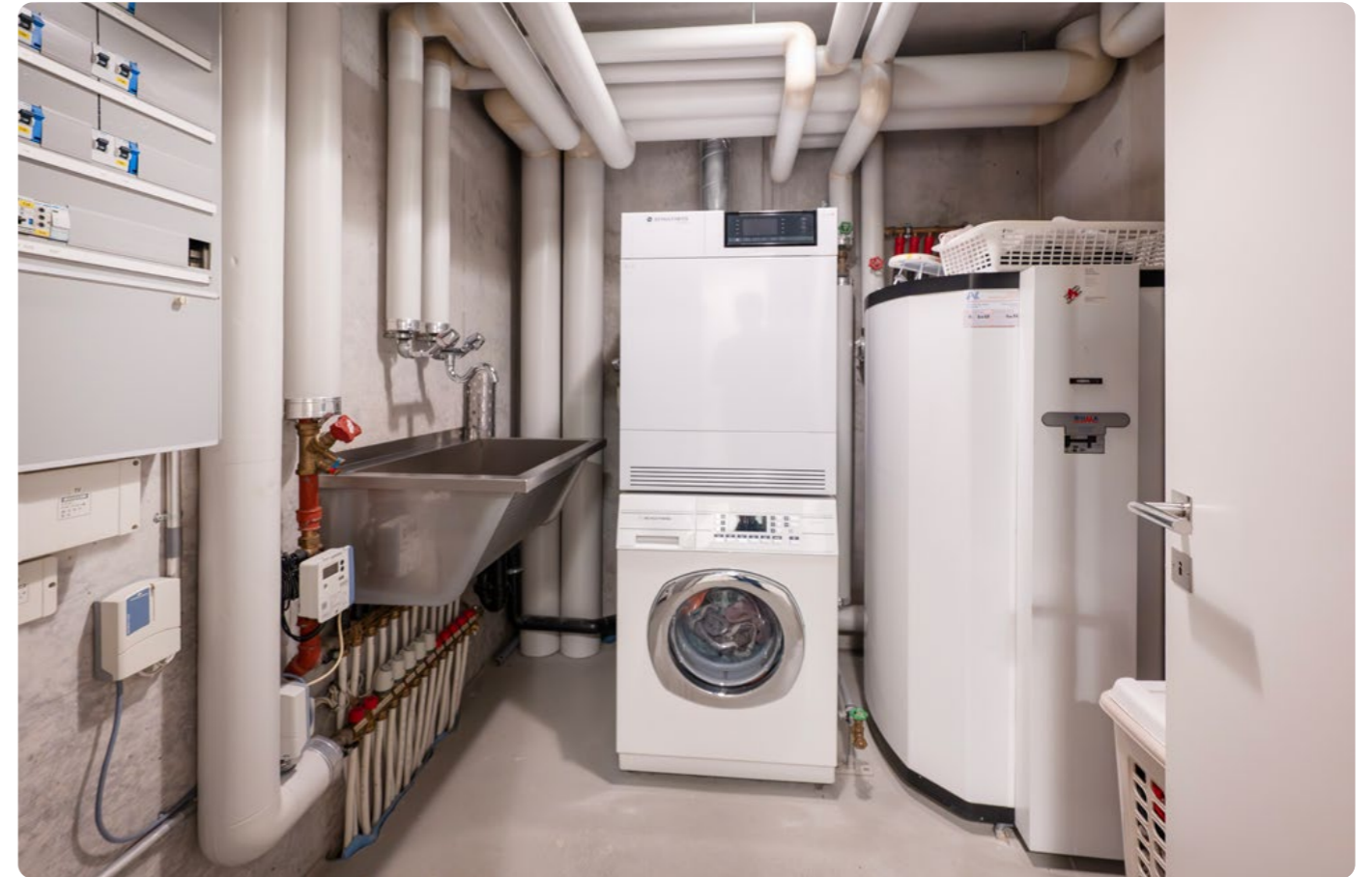
Laundry and Boiler room
